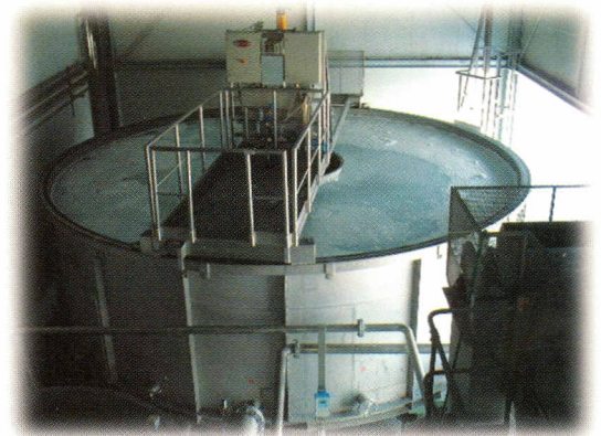
KLC 24 - Process water treatment (textile industry)
